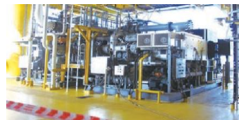
Vapor Recovery Compressor - Vietnam Offshore 3225MMC / 600kW
