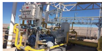
LPG Transfer Compressor - Mexico 6HK / 45kW
