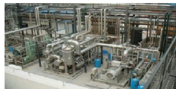
NH3 Recovery / Purification Plant - China 2520SSC / 280kW
