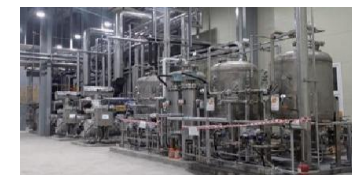
CO2 Liquefaction Plant - Korea 200S / 230kW
